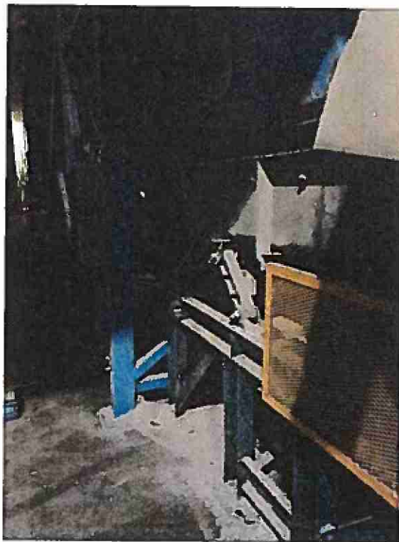
View of the crusher and a few inches of accumulated hazardous lead dust under the unit.
