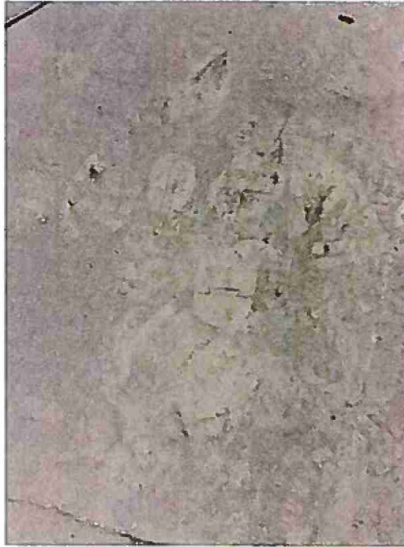
View of dust accumulation on the floor of the building.
